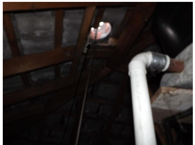
Hole in roof from previous chimney flue.
