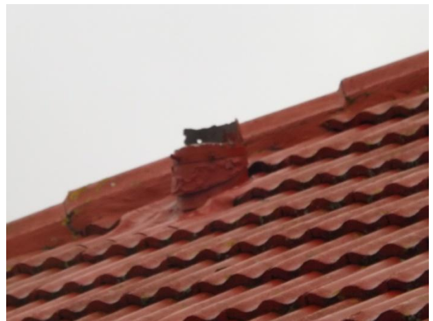
Hole in roof from previous chimney.
