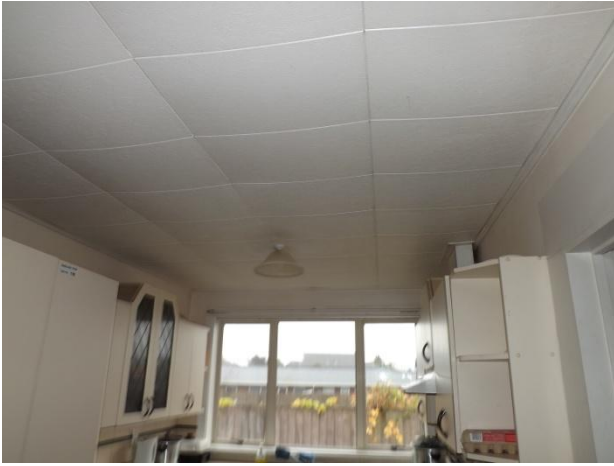
Kitchen ceiling tiles are sagging.
