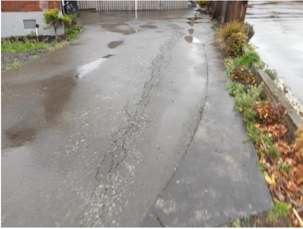
Slumping to tar-sealed driveway.
