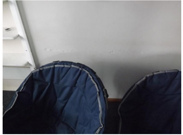
Dents in wall of lounge.
