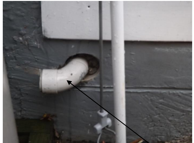
Not sure what this waste-pipe is for.
