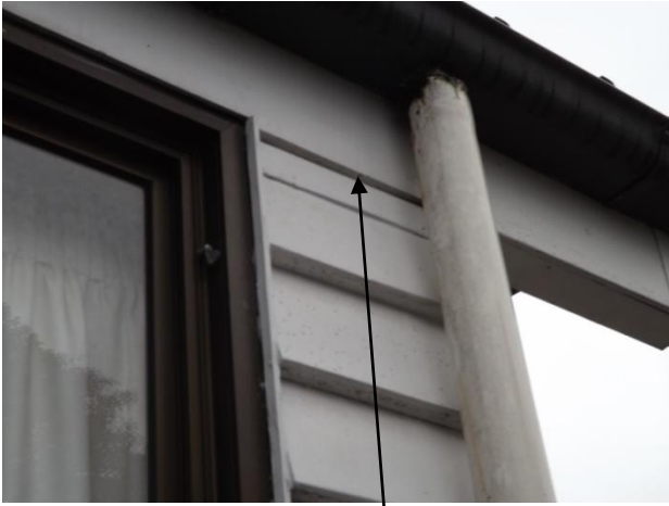
Small hole to cladding.
