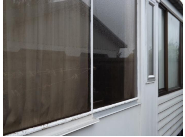
Two bedroom extension to east. Steel window beginning to rust.
