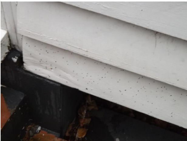
Rotten board and borer to east elevation.
