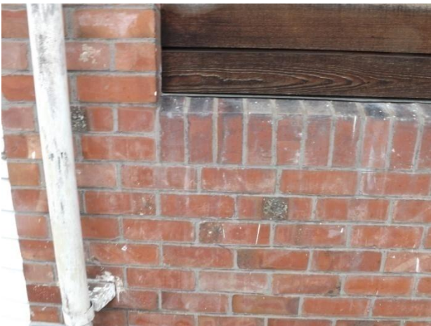
Very minor cracking to mortar-joints.
