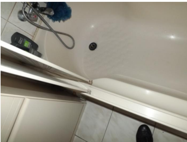
Screen-doors to bath not operating correctly.
