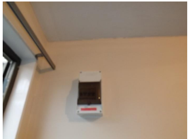
Sub-main to garage.
