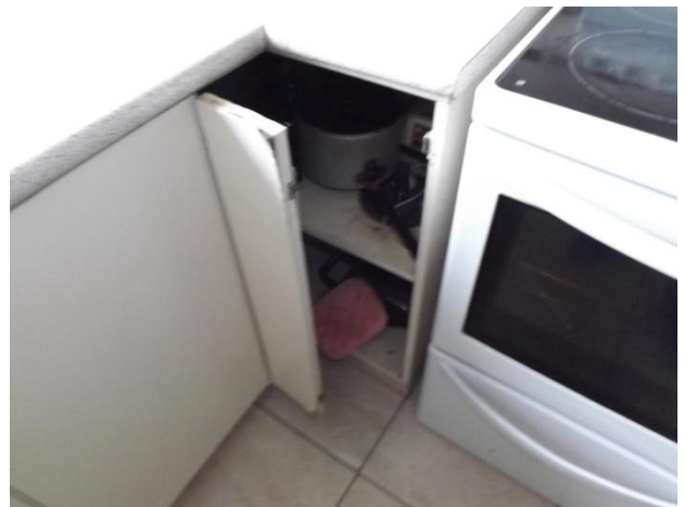
Loose door to kitchen units.
