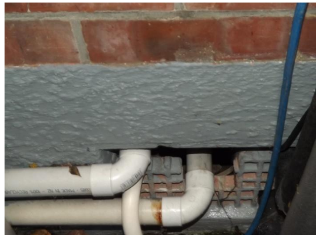
Holes around waste-pipes should be plastered.
