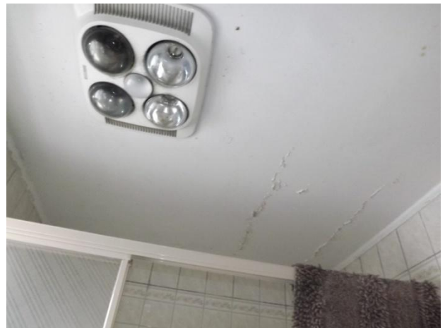
Paint deteriorating to bathroom ceiling.
