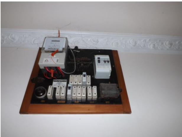
Switch board in good order; cloth mains cable.
