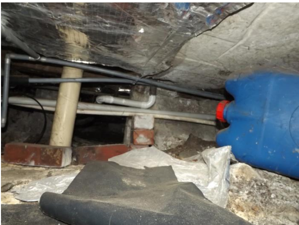
Galvanised piping and PVC waste-pipes.
