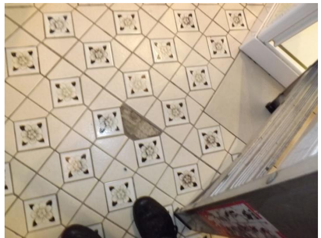
Tiles missing to bathroom floor.
