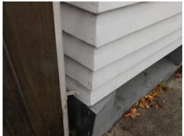
Borer to weather-boards.
