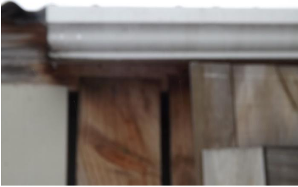
Water runs off the end of the lean-to roofing spouting.
