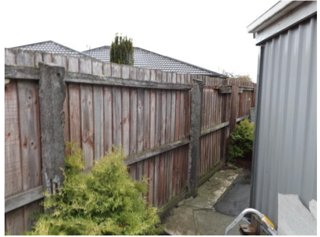
Deteriorating fence rails.
