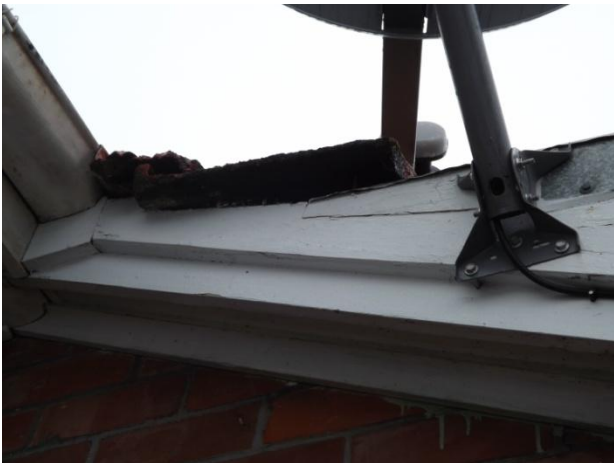
Hole in barge capping may allow south/ west rain inside.
